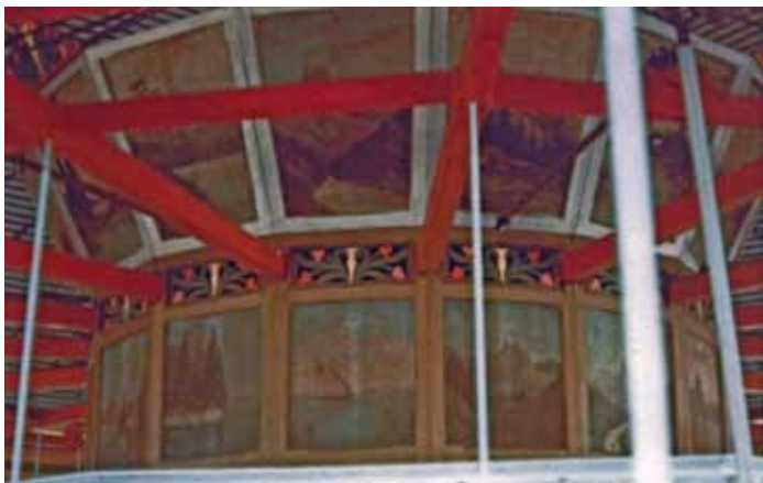
Inner housing of Marshall Hall carousel showing original artwork. Courtesy of Gray Tuttle.
